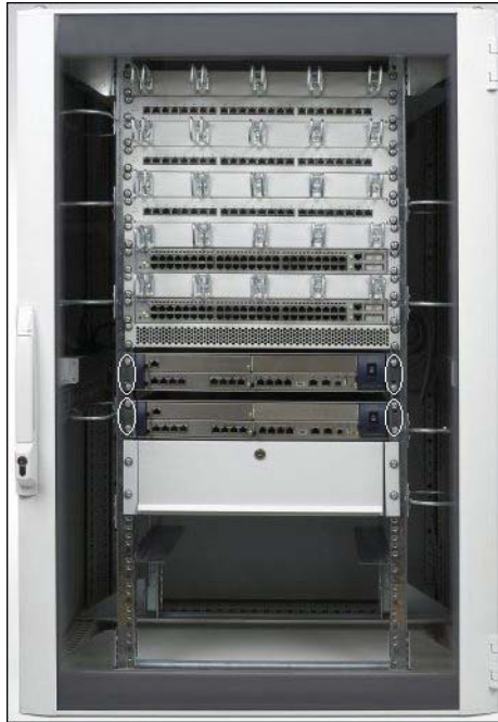
Figure: Two OpenScape Office MX system boxes in the 19" rack
